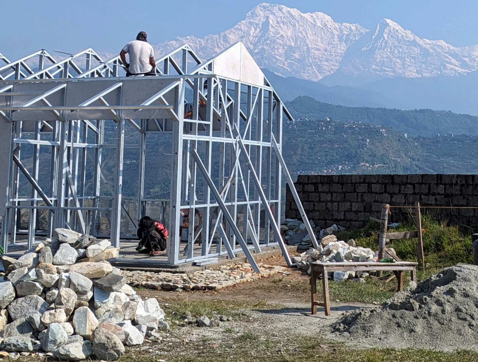
Building of double Earthquake Resilient Classrooms at Janasiddha Basic School in Harpan Village in Kaski District of Nepal.
